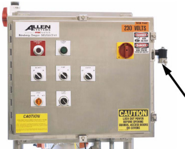
Figure 2-2 Circulation Solenoid Location
